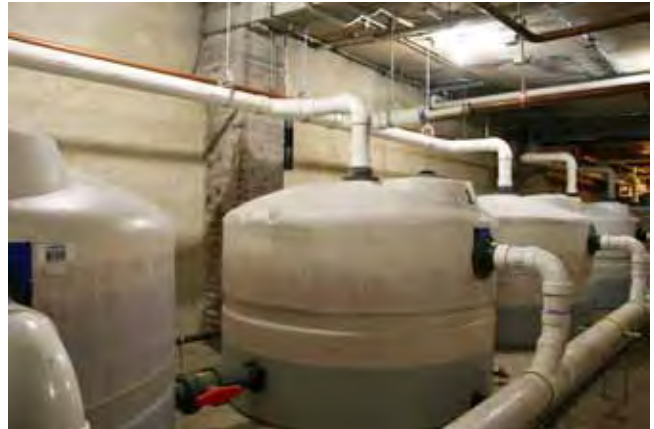
A few of the 660-gallon cisterns at Friends Center in Philadelphia, PA. These are a small part of the complex system that collects rainwater and reuses it throughout a newly renovated building. Photo by Lynn Alpert.
