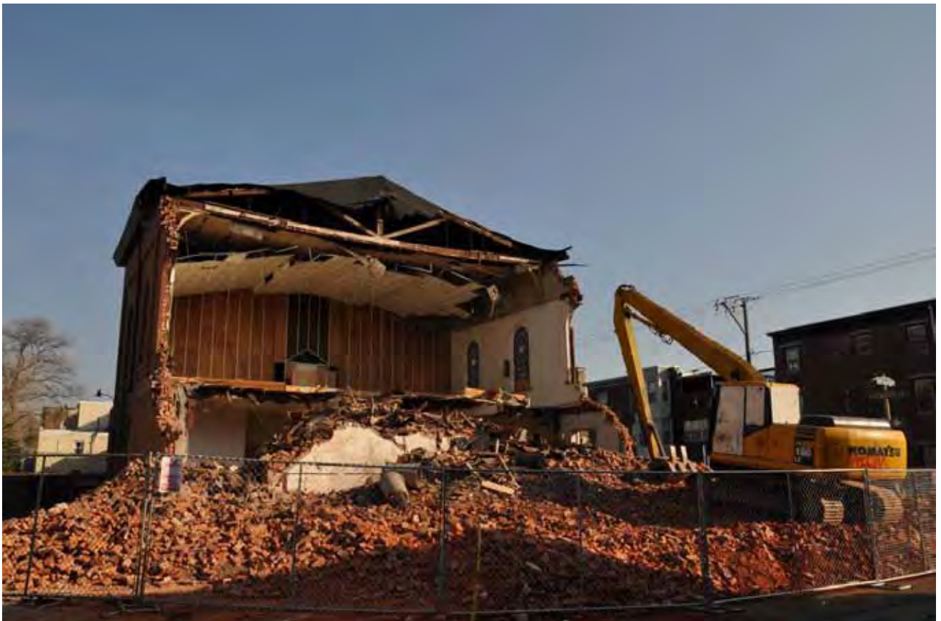
Philadelphia's Metropolitan AME Zion Church, built in 1861, was demolished in February 2011 to make way for construction of six new rowhouses. Photo courtesy of Laura Blanchard.
