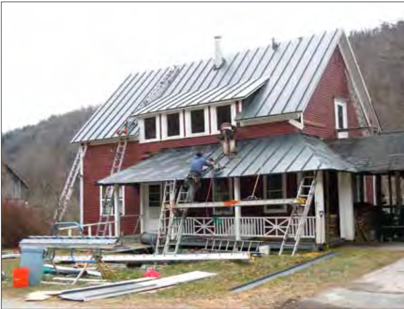
One of the many projects completed since the Church of Our Saviour went through New Dollars/New Partners training was putting a new roof on their guest residence, Heminway House. Photo credit: Anne Clarke Brown
